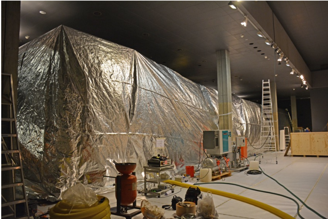
Figure 4 Bubble for anoxic treatment, the biggest one the contractor built so far
